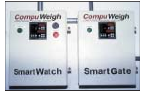
Control boxes for SmartWatch software package, which provides hazard monitoring for legs and conveyors, and SmartGate software, which controls the operation of 10 actuator gates for on-the-go blending during loadout.
