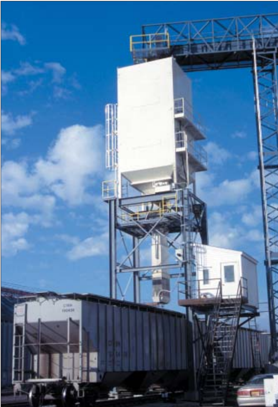
New 60,000-bph bulk weigh loadout scale is under the control of a CompuWeigh GMS 4000 package, which interfaces with a PC controller in a loadout shed shown below right of the scale.
