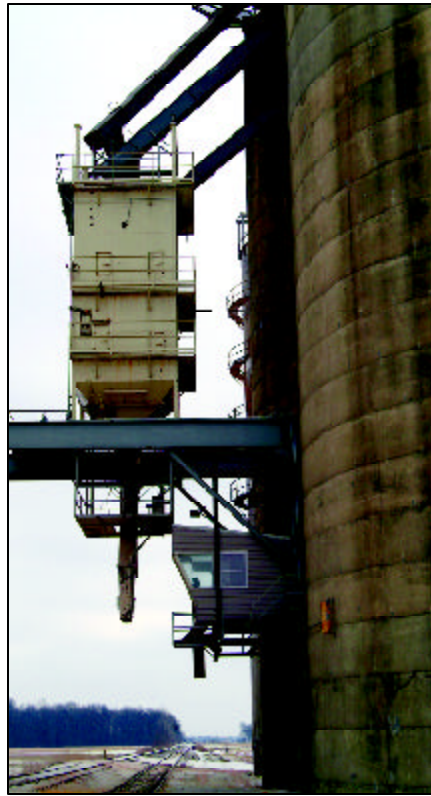
New 60,000-bph CompuWeigh bulk weigh loadout scale allows Kokomo Grain to load 85-car unit trains on the Norfolk Southern.
