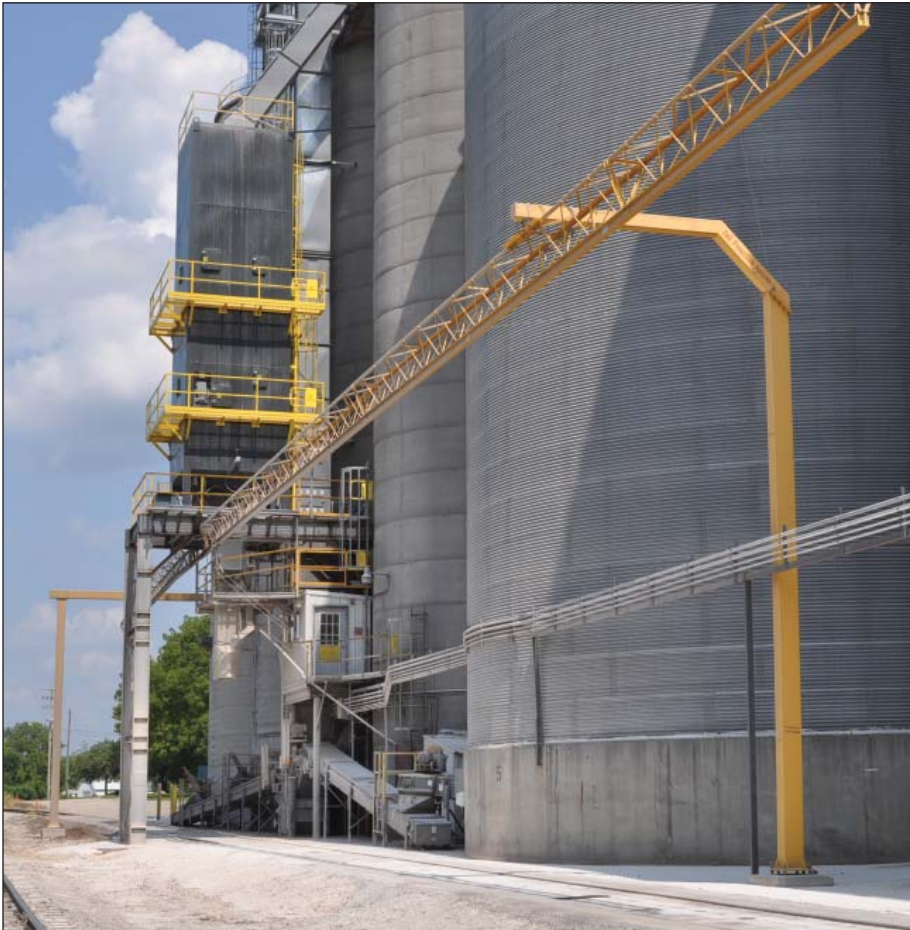
The new 60,000-bph, fully automated CompuWeigh bulk weigh loadout scale at The Andersons grain elevator in Reading, MI, installed the second week of July 2013 designed to load 75-car trains on the Indiana Northern short-line. Photos by Ed Zdrojewski.
