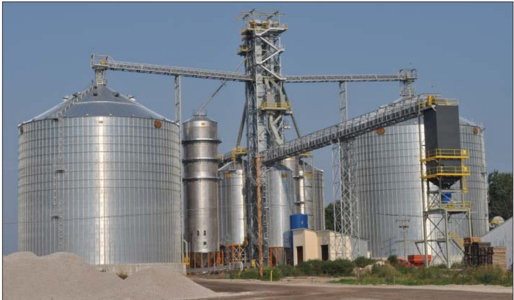
Auburn Bean & Grain Co.'s new 1.75-million-bushel rail-loading elevator at the edge of Standish, MI including two 730,000-bushel GSI tanks, two GSI grain dryers, and a 40,000-bph CompuWeigh bulkweigher. Photos by Ed Zdrojewski.
