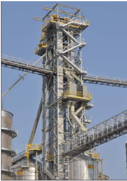
Closeup of the facility's LeMar center tower including 40,000- and 20,000-bph GSI legs, five-hole Hayes & Stolz rotary double distributor, and a pair of Magik Kleener gravity screeners.
