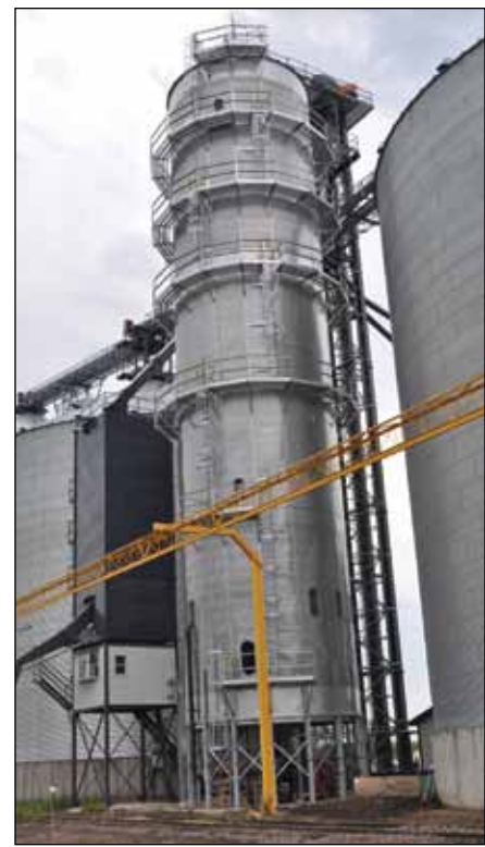
New 7,000-bph Zimmerman tower dryer, 30,000-bph bulk weigh loadout scale fabricated by J&D Construction, and trolley unit from Fall Protection Systems.
