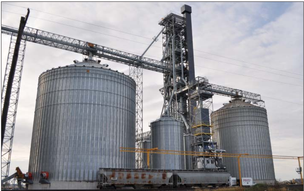
Closeup view of the newest construction at the Milmine elevator, including five corrugated steel tanks, four legs, a tower dryer, and bulk weigh loadout system for origin weights. Ground level photos by Ed Zdrojewski.
