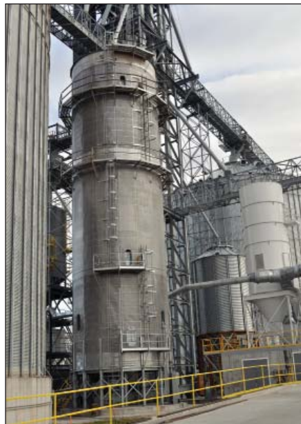
New natural-gas-fired 5,000-bph Zimmerman tower dryer in foreground and AIRLAN-CO baghouse dust control system to the rear.
