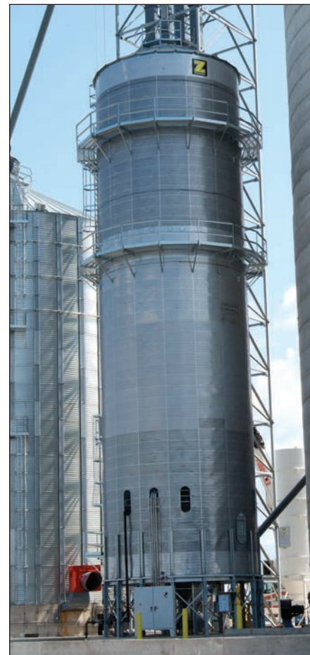
LP-gas Zimmerman tower dryer has the capacity to dry 5,000 bph of grain at five points of moisture removal.
