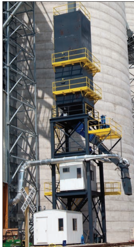
CompuWeigh bulk weigh loadout scale is designed to load a shuttle train, under normal conditions, in less than 10 hours. Ground level photos by Ed Zdrojewski.
