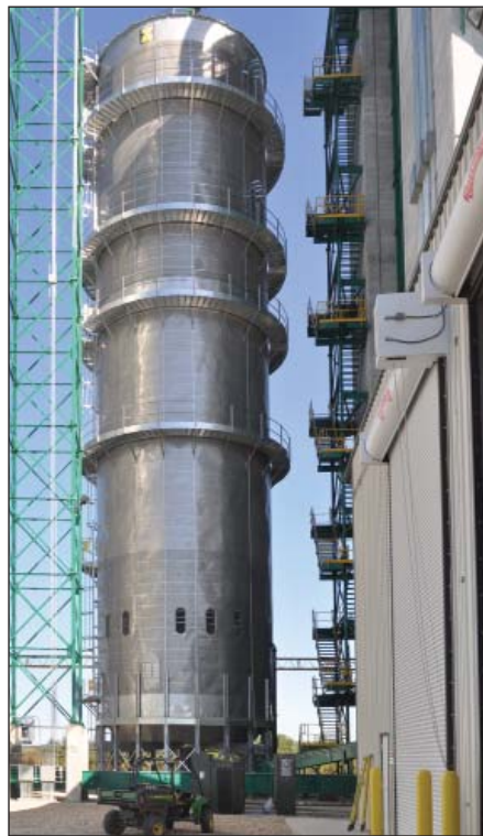
New Zimmerman 10,000-bph tower dryer is powered by natural gas from a new pipeline running out from town.
