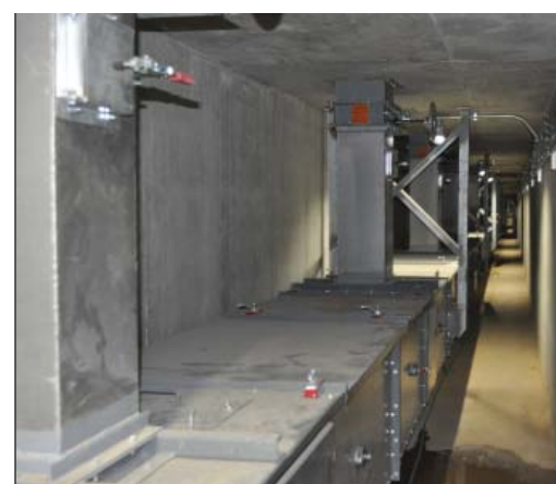
Hi Roller 20,000-bph enclosed reclaim belt conveyor in below-ground tunnel.
