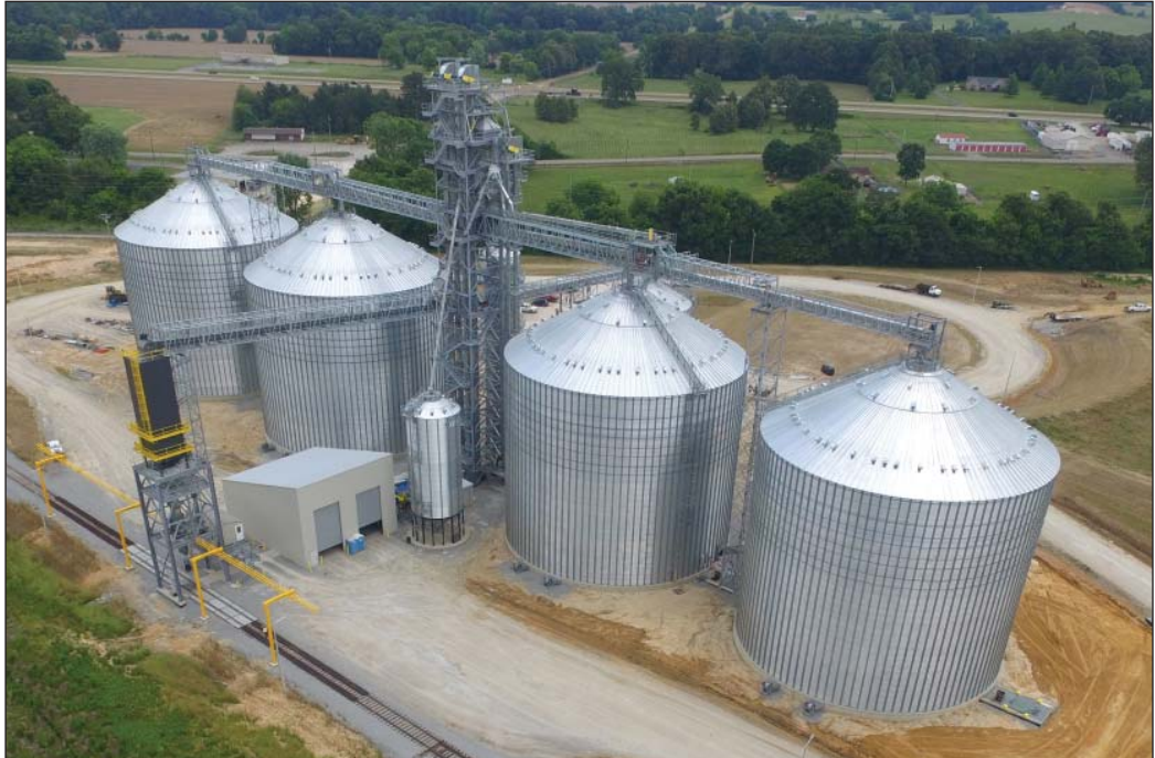
The Andersons' Inc.'s new 2.9-million-bushel rail terminal nearly complete north of Humboldt, TN. Aerial drone photo courtesy of ASM Engineering Consultants, LLC.
