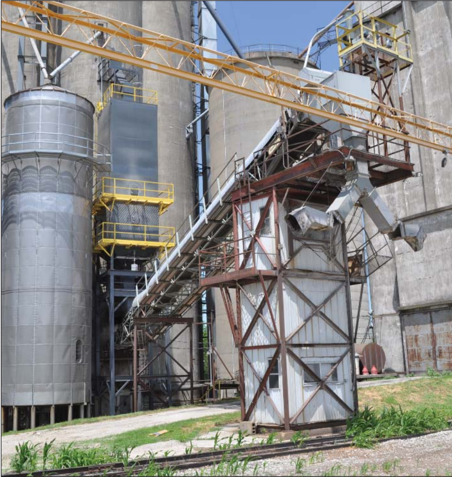
Farmers Grain Co. of Central Illinois installed a new CompuWeigh 30,000-bph bulk weigh loadout scale, shown at left, under the control of a CompuWeigh GMS 4000 automation system, at Chestnut, IL. Photo by Ed Zdrojewski.
