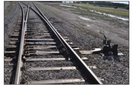
Loop track rails, laid by R&R Contracting, are stapled to high-carbon steel ties.
