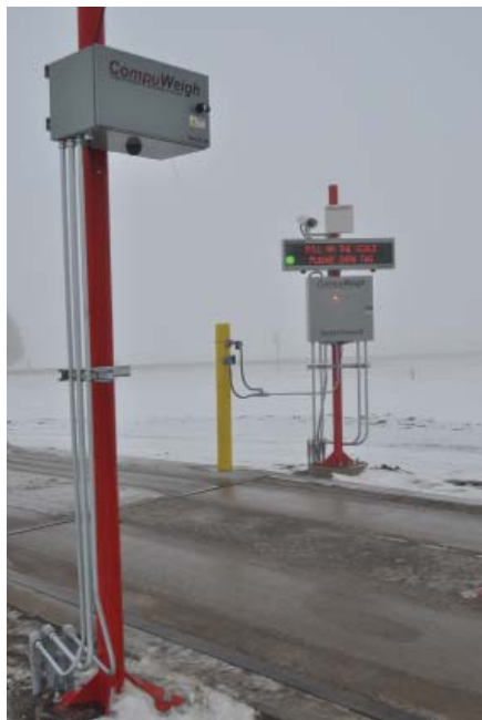
New CompuWeigh RFID card reader and SmartView display board installed alongside the new inbound scale. Photo by Ed Zdrojewski.
