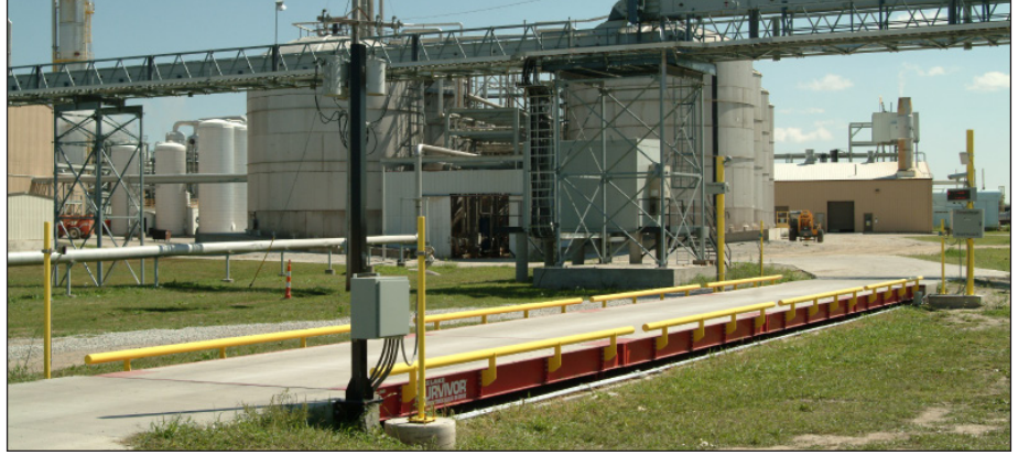
New Rice Lake Weighing Systems truck scales, with a streamlined accounting system from Intelligo and an automated truck management system from CompuWeigh, have been installed by Aventine at Aurora West and NELLC.
