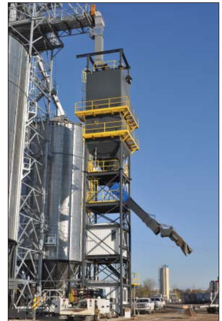
New 50,000-bph CompuWeigh bulk weigh loadout scale is designed for loading both containers and covered hopper railcars. Brock 40,000-bushel hopper tank is visible to the left of the bulkweigher.
